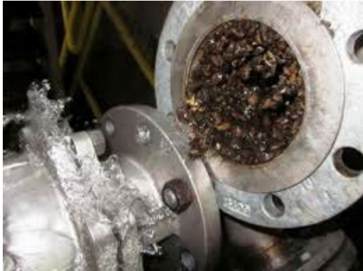
A three-foot-diameter pipe clogged by zebra mussels in less than three months (U.S. Department of Energy)
