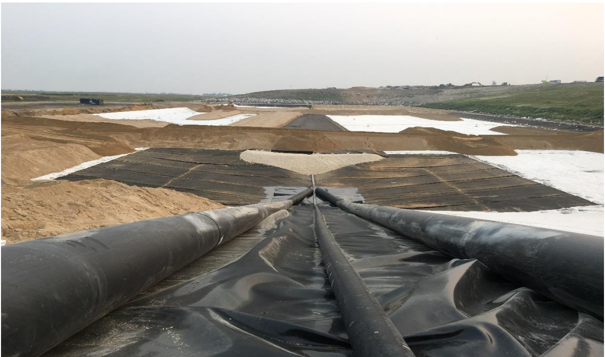
Leachate Collection pipes in Sump
