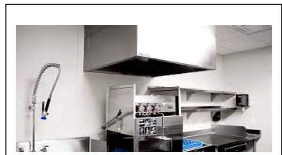
Figure 8: Type II Condensate Hood in Dishwasher Area.
