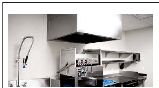
Figure 8: Type II Condensate Hood in Dishwasher Area.
