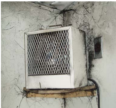
Incorrect placement: heater's air exhaust is obstructed.
