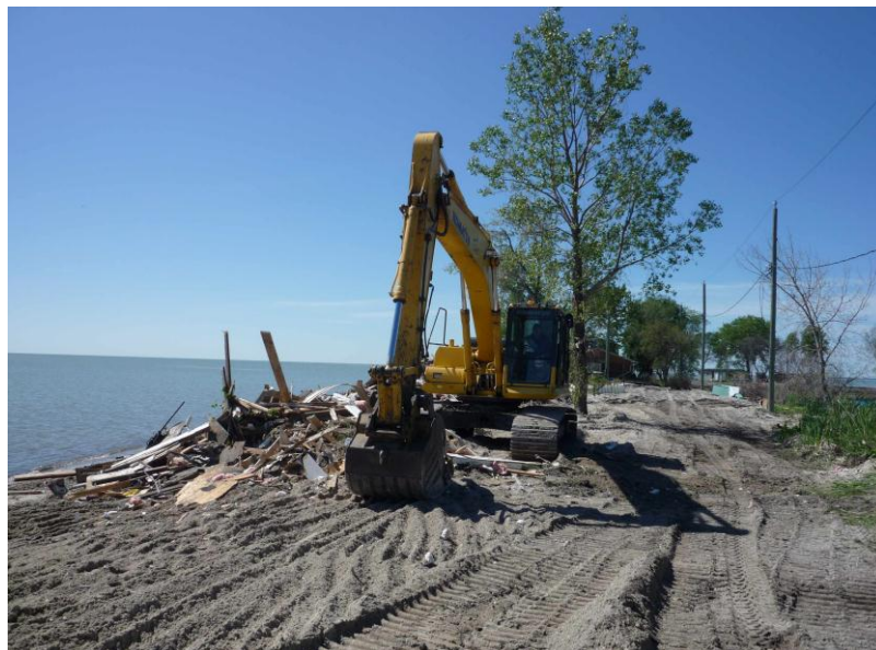
Damage due to Flooding at Big Point near Langruth
