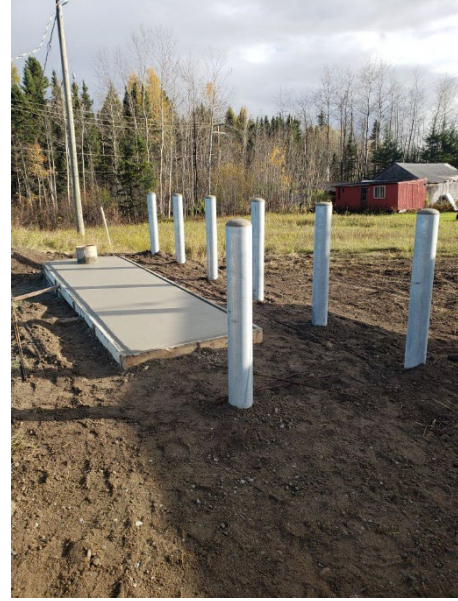
Wabowden Water Treatment Plant Generator
