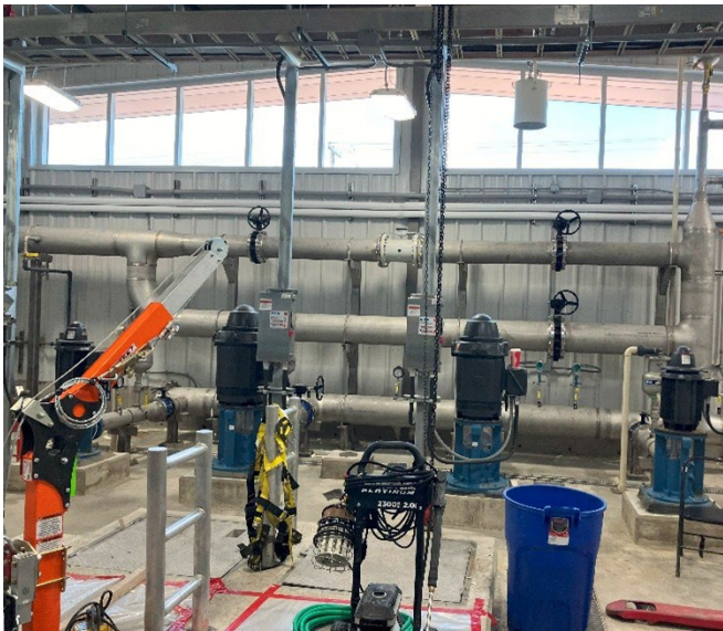
Town of Beausejour Water Treatment Plant
