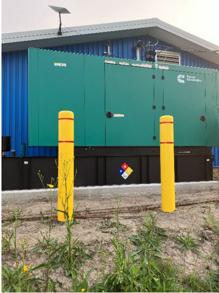
Wabowden Water Treatment Plant Generator
