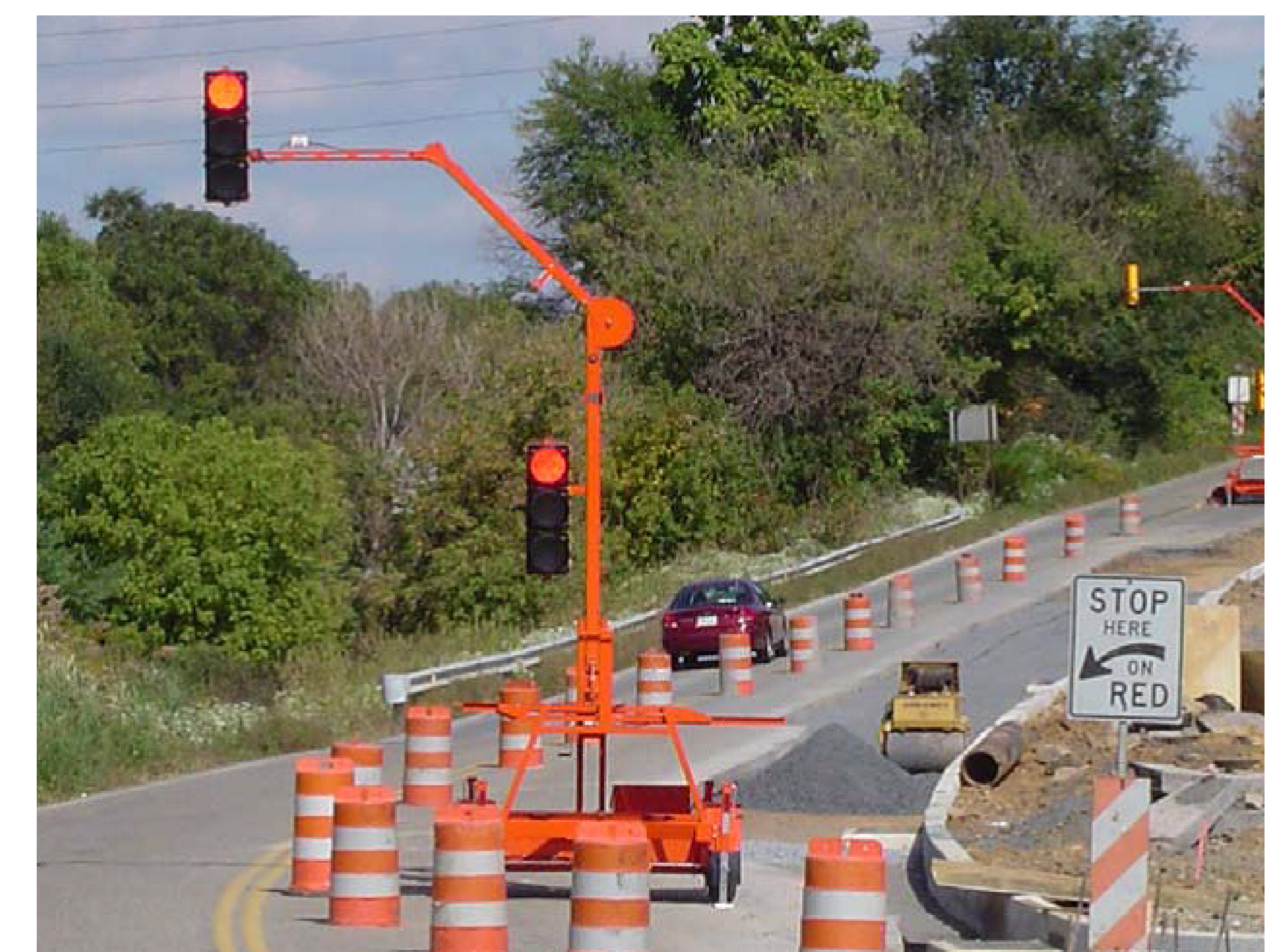
Above: Example of single lane with signal light control
