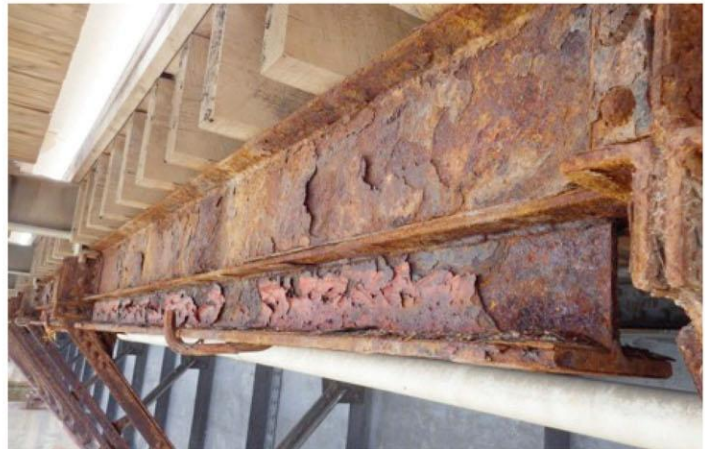
The northerly edge beam is severely deteriorated.
