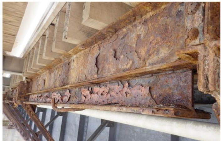
The northerly edge beam is severely deteriorated.
