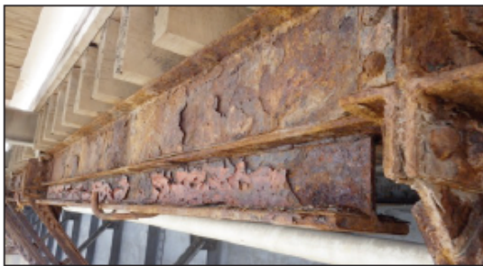
Severe deterioration of the edge beam on north side.
