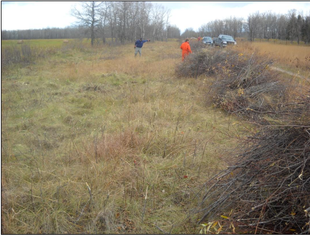
Figure 8. Brush clearing at the south Interlake trail site where shrub encroachment had been identified as a threat to Small white lady's-slippers growing at this site.
