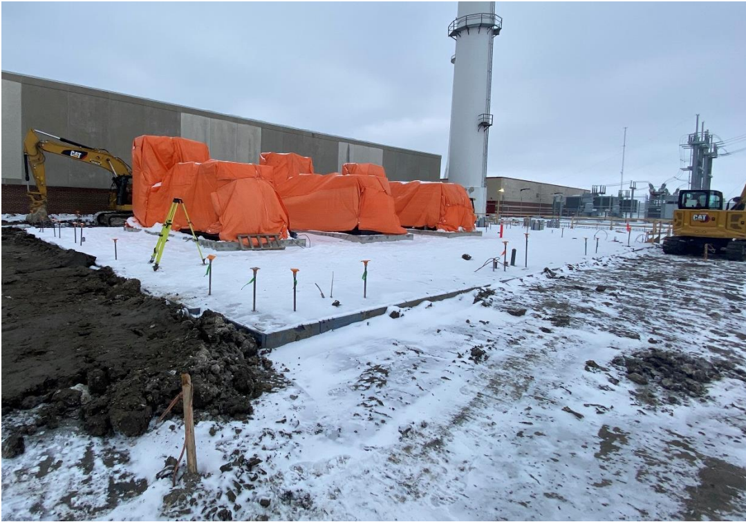
Figure 3: Standby Generator Building
