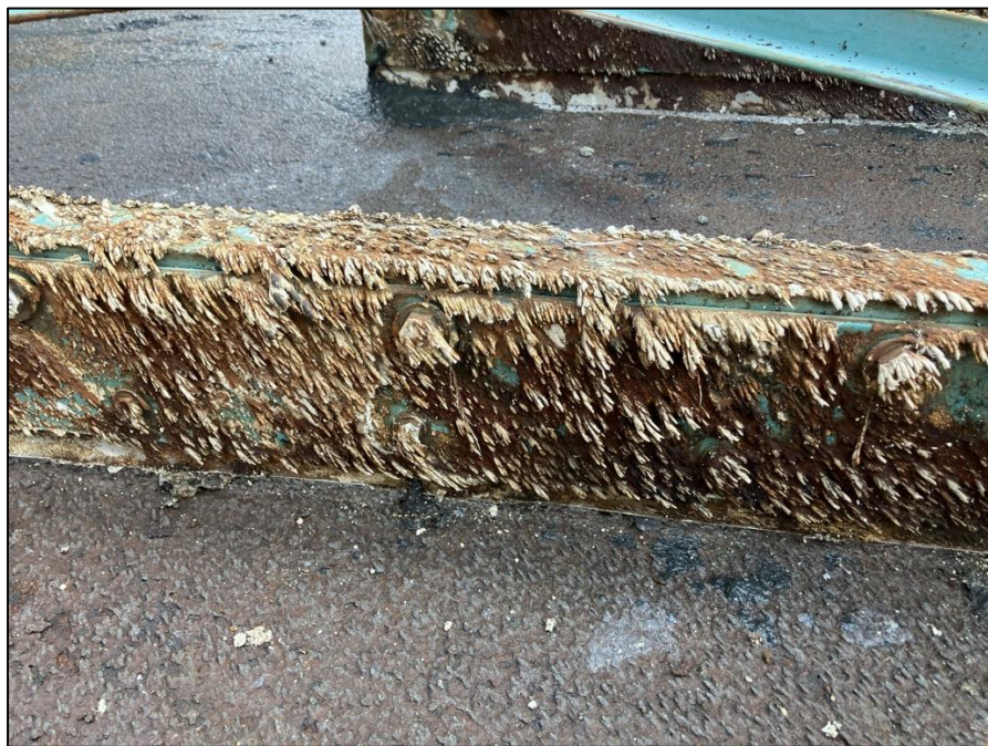
Figure 7: Ferric Deposits on Primary Clarifiers
