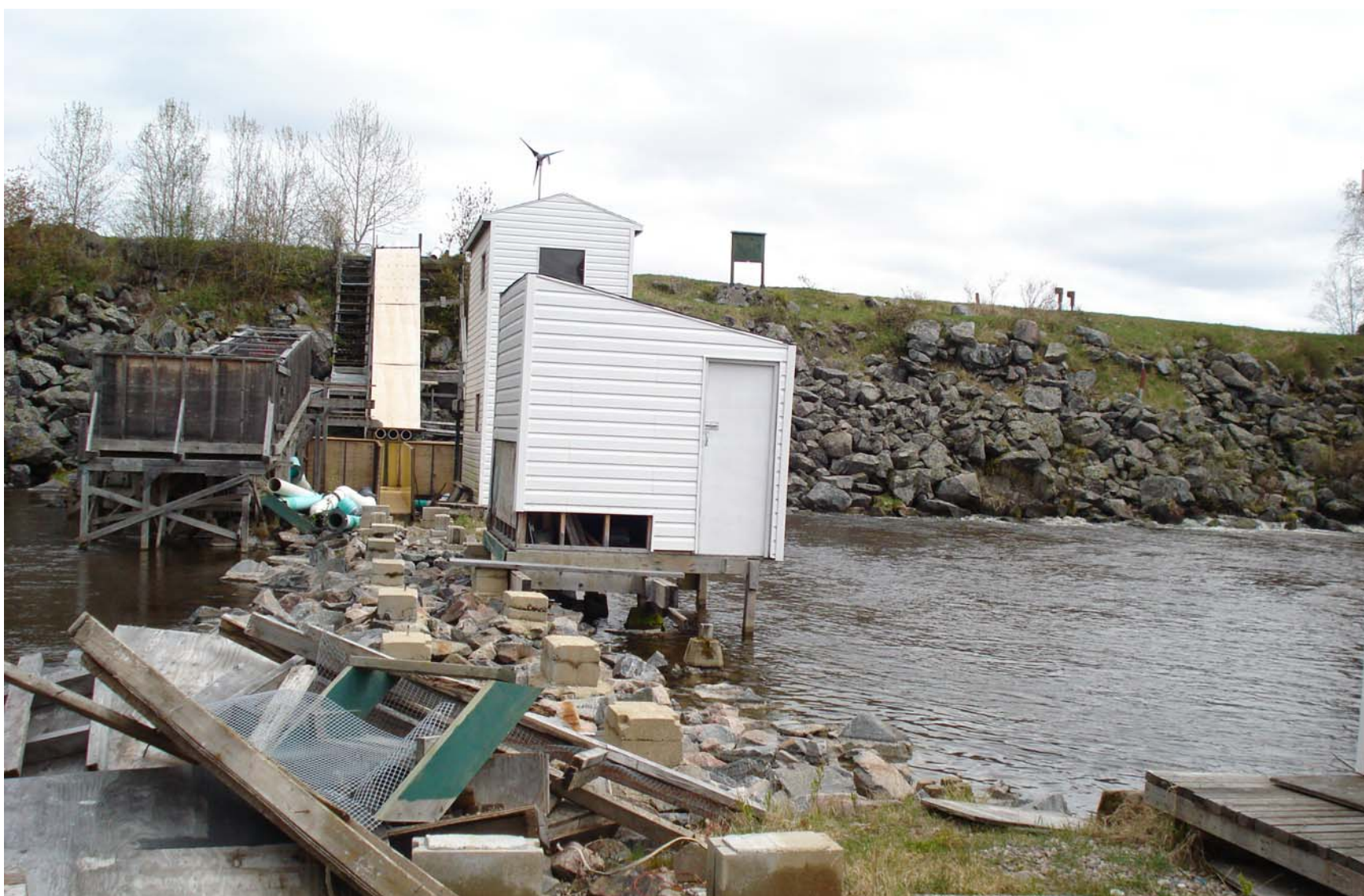
Figure 4. Photograph of the upstream face of the Pinawa Diversion Dam, showing the existing fish study structure slated to be removed before remediation of the Dam begins.
