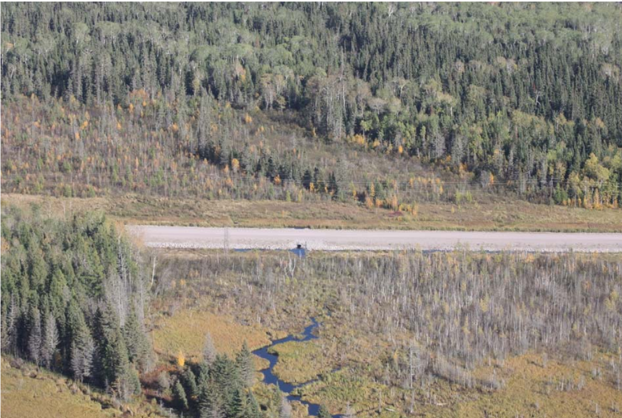
Photo 14: Small drainage/stream crossing – single culvert (representative from P1) Photo Credit: Joro Consultants
