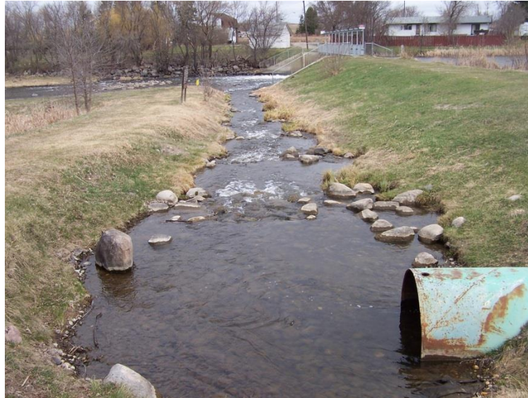
Figure A5-1. View of the pool and riffle structure of the Rapid City fish ladder, April 25, 2012.
