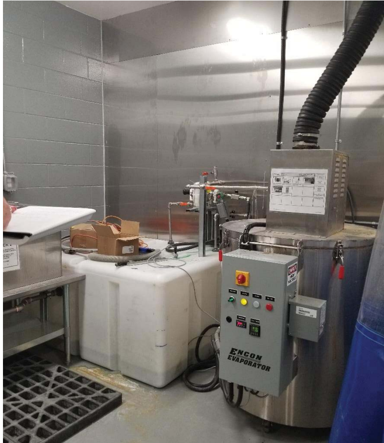
Photo B-2: EconDrum Evaporator and Alodine line rinsewater storage
