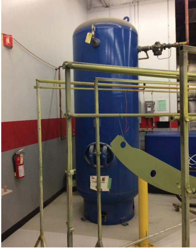
Photo B-15: Air compressor servicing the tools throughout the plant
