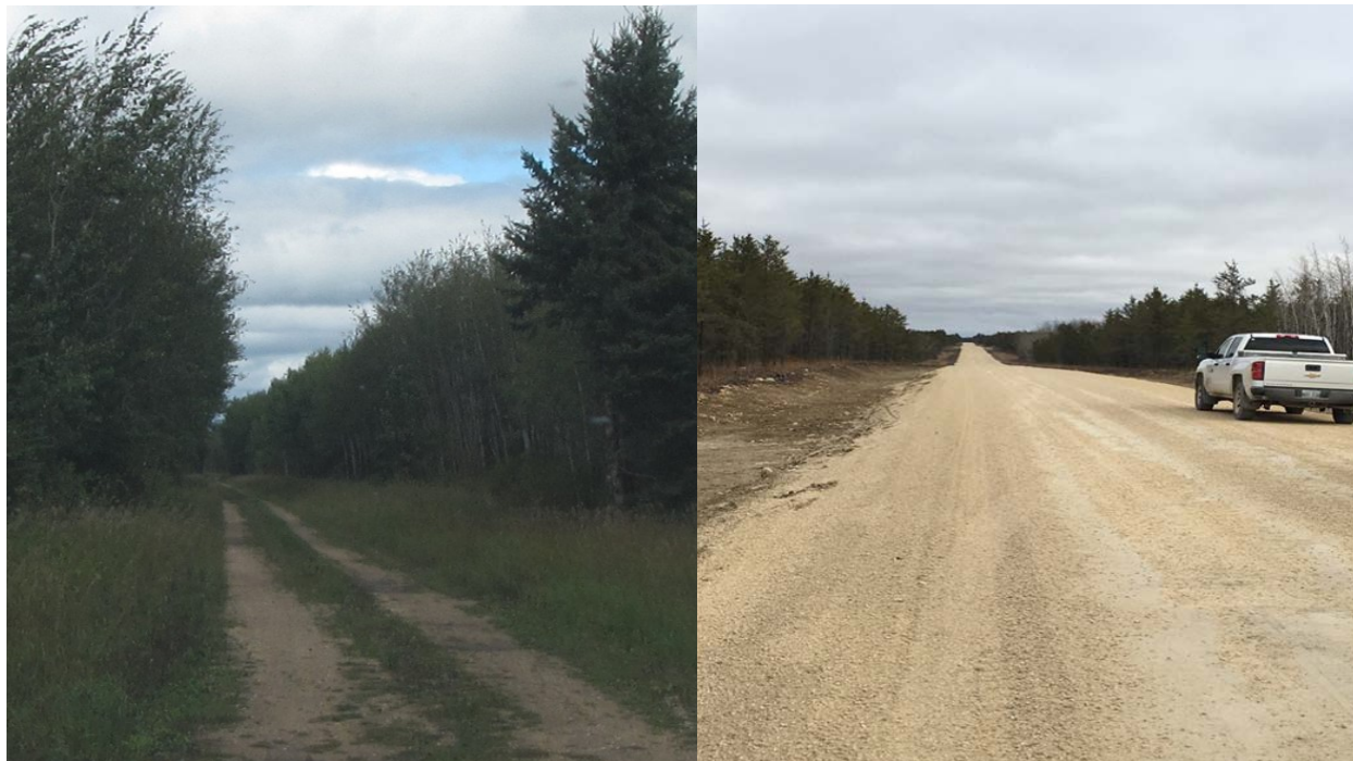
Photograph 2-2. Picture of the Forestry (Idylwild) Road: Prior to Construction in 2016 (left); and after Construction in 2018 (right)
