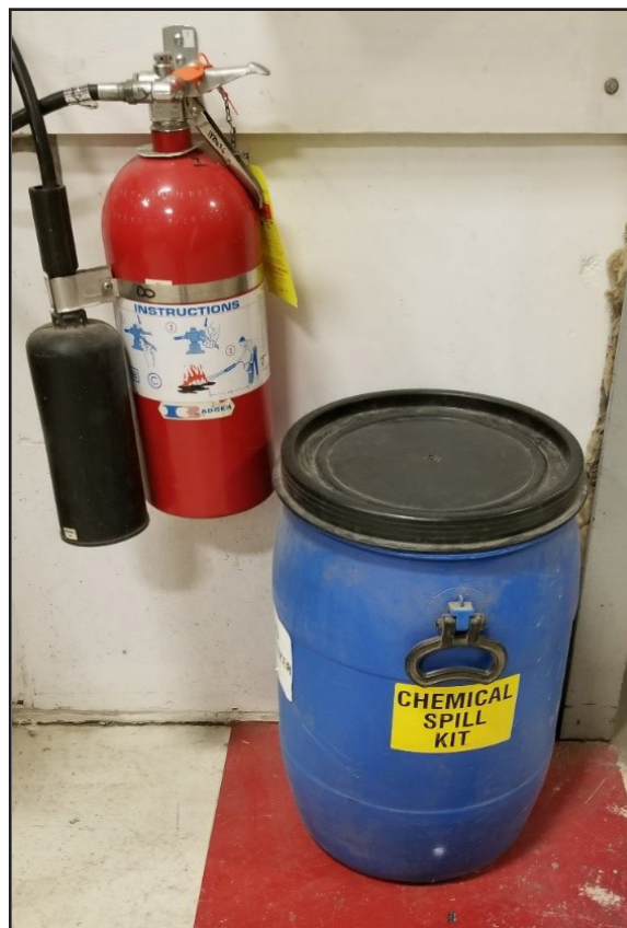
Photo B-5: Example of a chemical spill kit and fire extinguisher, located in the warehouse area.
