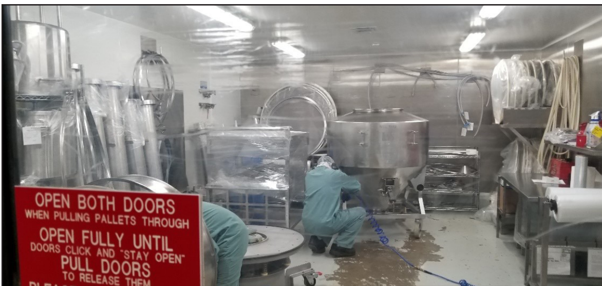
Photo B-27: Parts drying area showing compressed air hoses.
