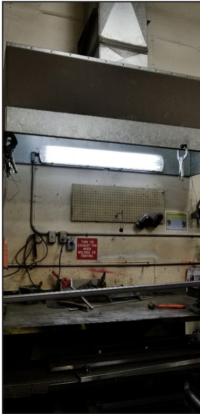
Photo B-14: Maintenance shop fume hood and work bench for welding.
