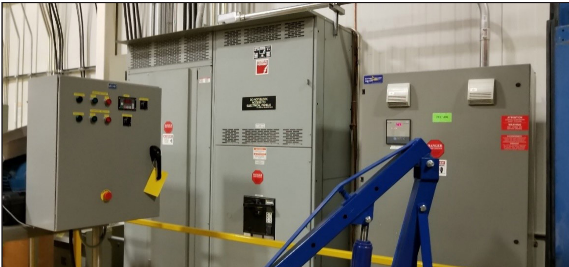
Photo B-7: Electrical panels on-site, located in the warehouse area.
