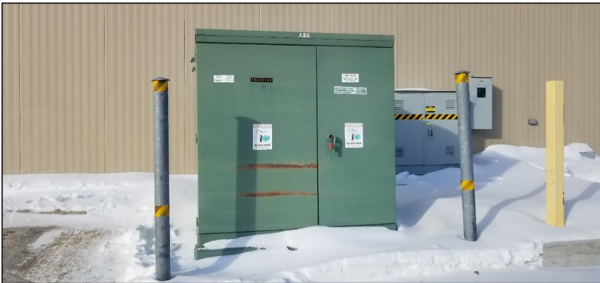
Photo B-23: Ground level transformer (PCB free) located on the east side of the plant.
