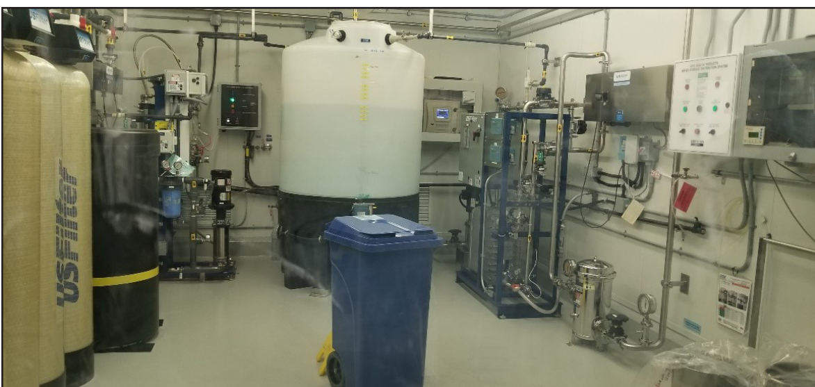
Photo B-9: Purified water room, located in the manufacturing area, showing reverse osmosis system.
