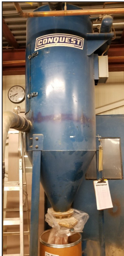
Photo B-17: Dust collector in the mezzanine, showing fiber drum collection system.
