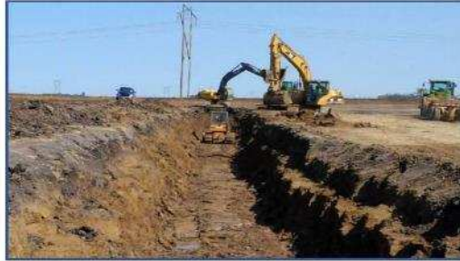
Figure 5. Construction of an engineered seepage cut-off trench on a water storage reservoir (PBS Water Engineering Ltd.).
