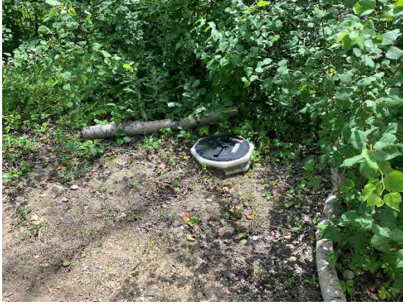
1.1 Typical Underground Wastewater Holding Tank
