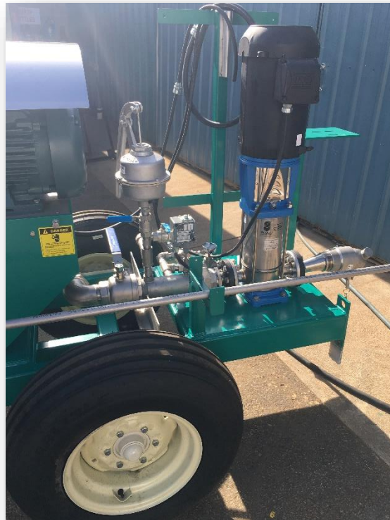
Figure 4 - Pump Package Visual
