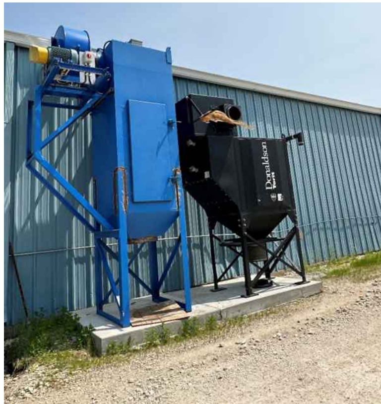
Photo 24: General view of bag house filtration system associated with the welding area. (Tetra Tech, June 2023)
