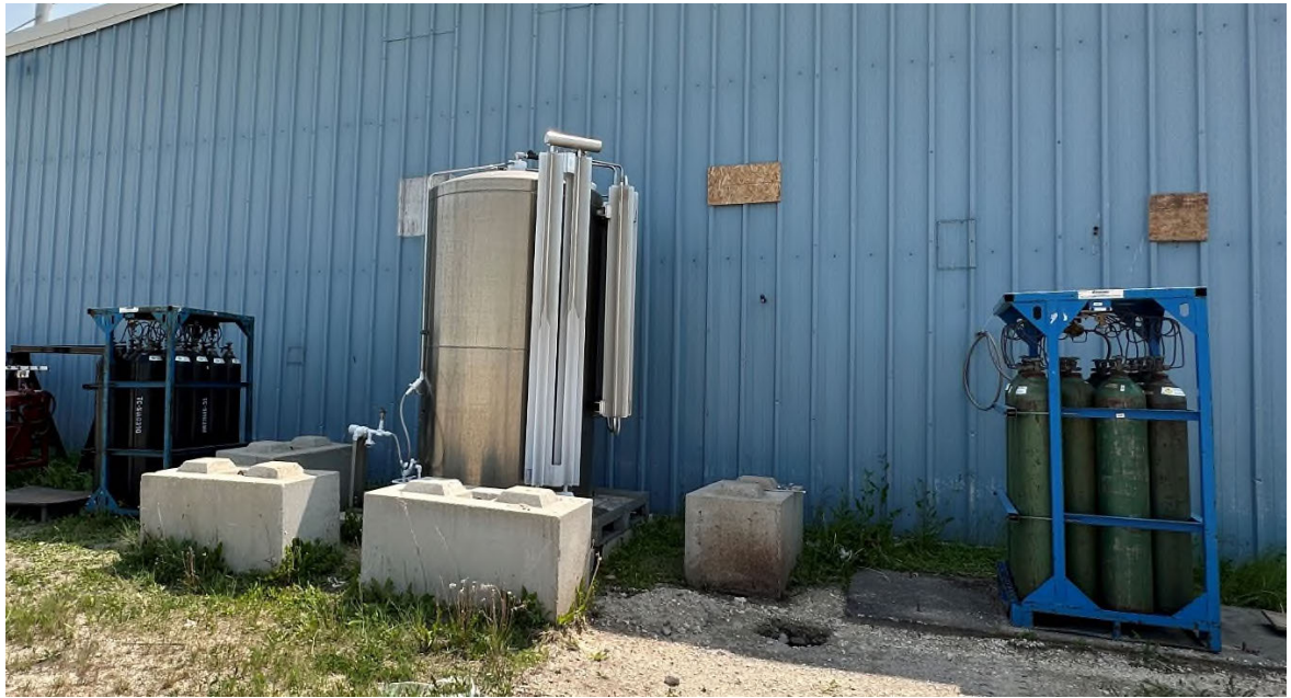
Photo 23: General view of microbulk nitrogen tank and associated compressed gas cylinders. (Tetra Tech, June 2023)
