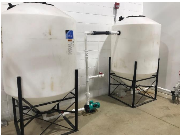
Photo 8: New inhouse wastewater processing equipment. Wastewater will be put into the first tank and ferrous sulphate will be added and agitated. Sodium hydroxide will then be added and resulting pH is around 9. Allow to settle and then filter to get to a pH of between 6-8. Carbon treated prior to release if required. Very little sludge is generated, and the filter would be periodically inspected to remove any accumulations.
