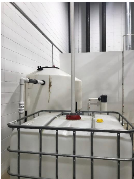
Photo 9: New inhouse wastewater processing equipment
