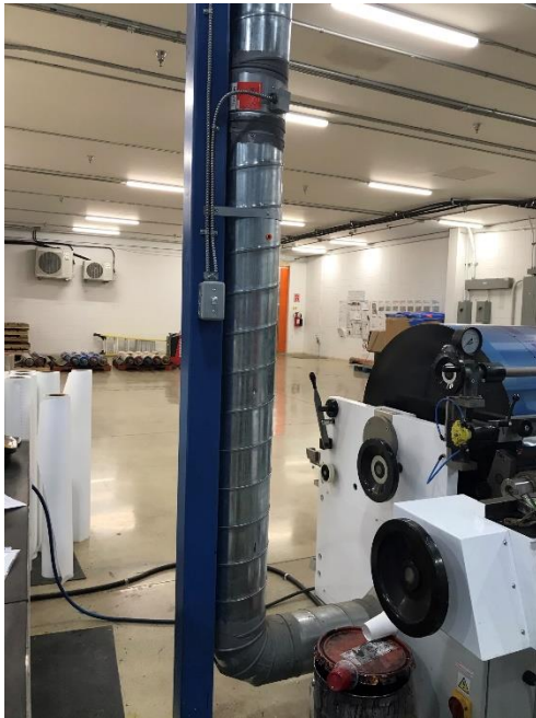
Photo 12: Proofing press exhaust is vented up and out of the roof and only operational when press is running.
