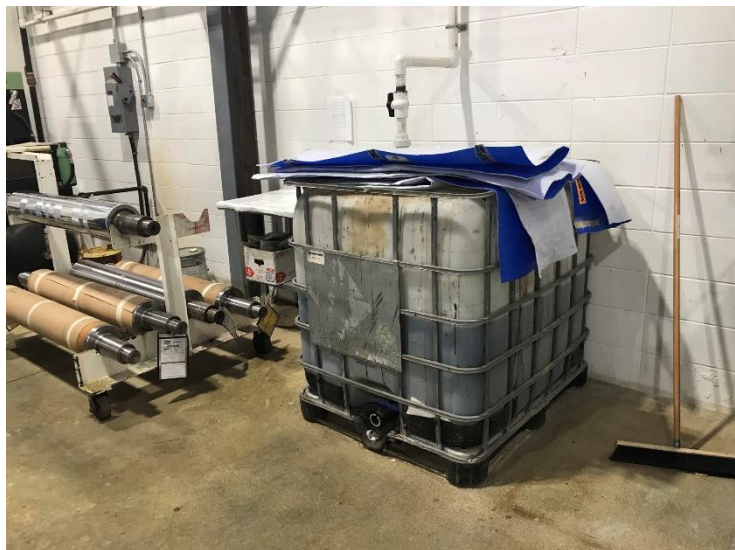
Photo 5: Chromic Wastewater Tote - wastewater is piped into the tote via overhead piping. Totes are emptied by Miller Environmental approximately twice a year as limited amount of chromic wastewater is generated due to the water being recycled and reused during operations.
