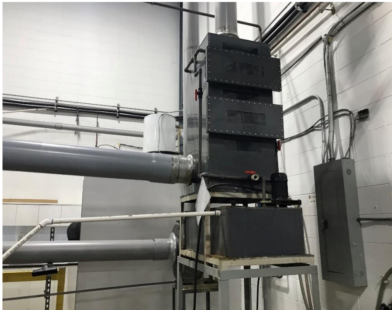
Photo 1: Chrome tank scrubber with venting to roof
