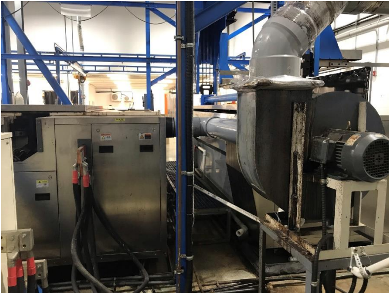
Photo 2: Chrome tank with venting
