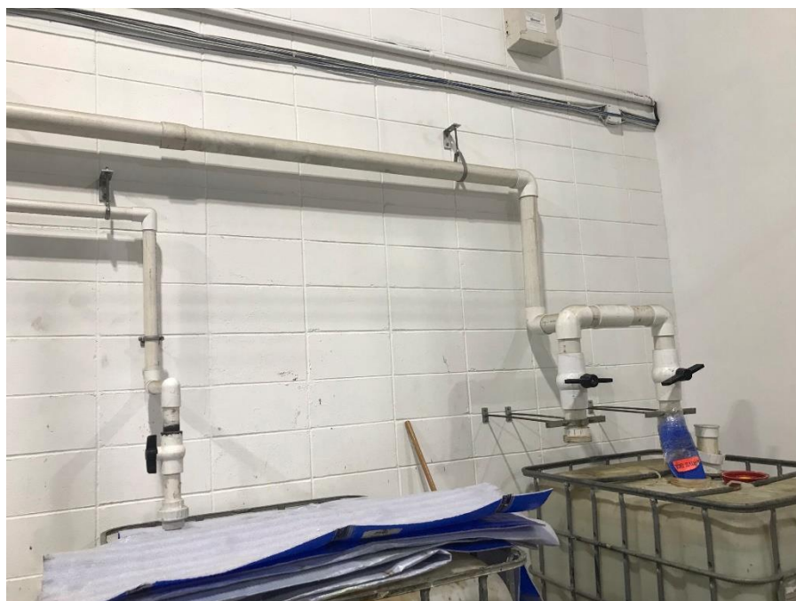
Photo 7: Overhead piping for moving wastewater from the three tanks (nickel, copper, and chromium) to holding totes.
