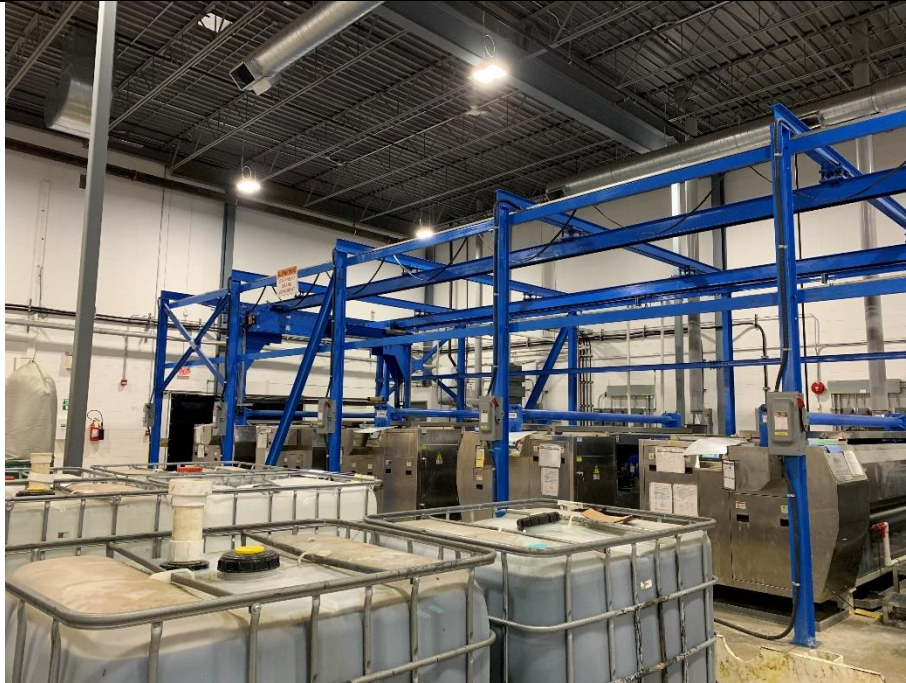
PHOTOGRAPH 3: Hazardous wastewater stored in 1000 L totes, prior to being pumped by Miller Environmental.
