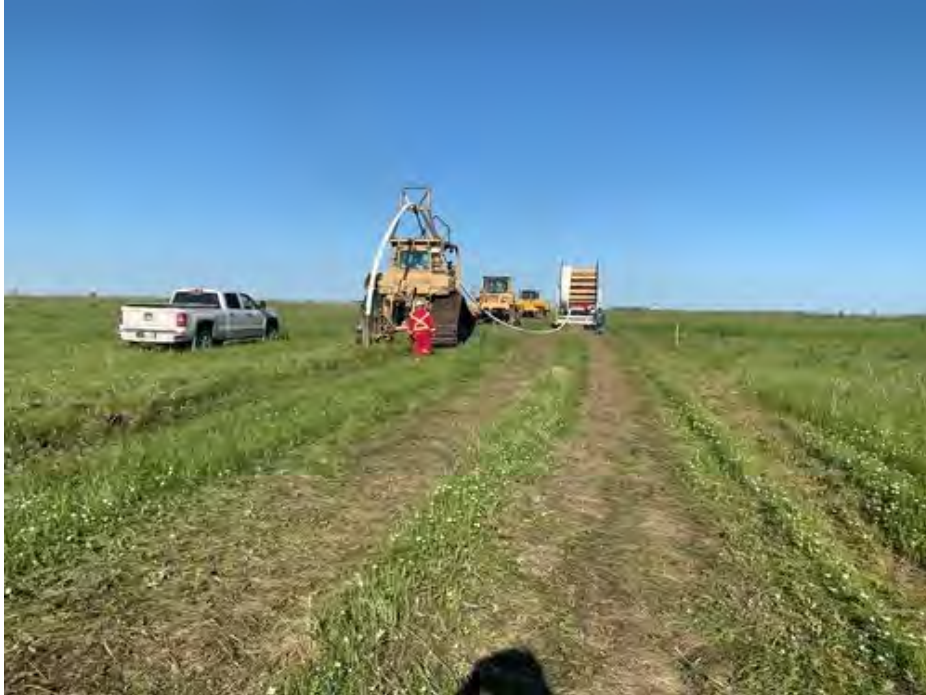
107. Example photos only. Not photograph of current project - Spoolable composite flowline conduit, un-reeling flowline conduit in preparation for placement in ploughed trench.
