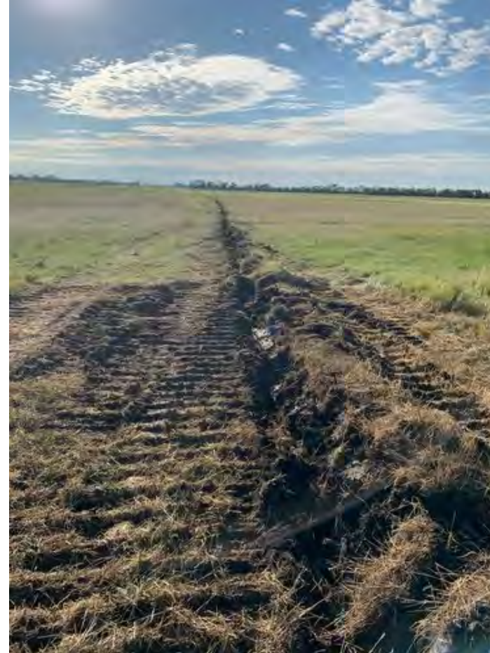
108. Example photograph only. Not photos of current project. Minimally disturbed flowline trench immediately after flowline installation.
