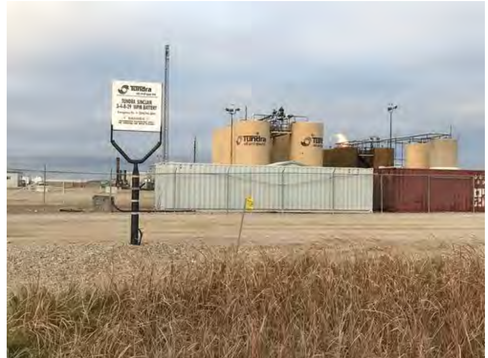
106. Looking north at Tundra Sinclair 03-04-008-29 W1M battery site.
