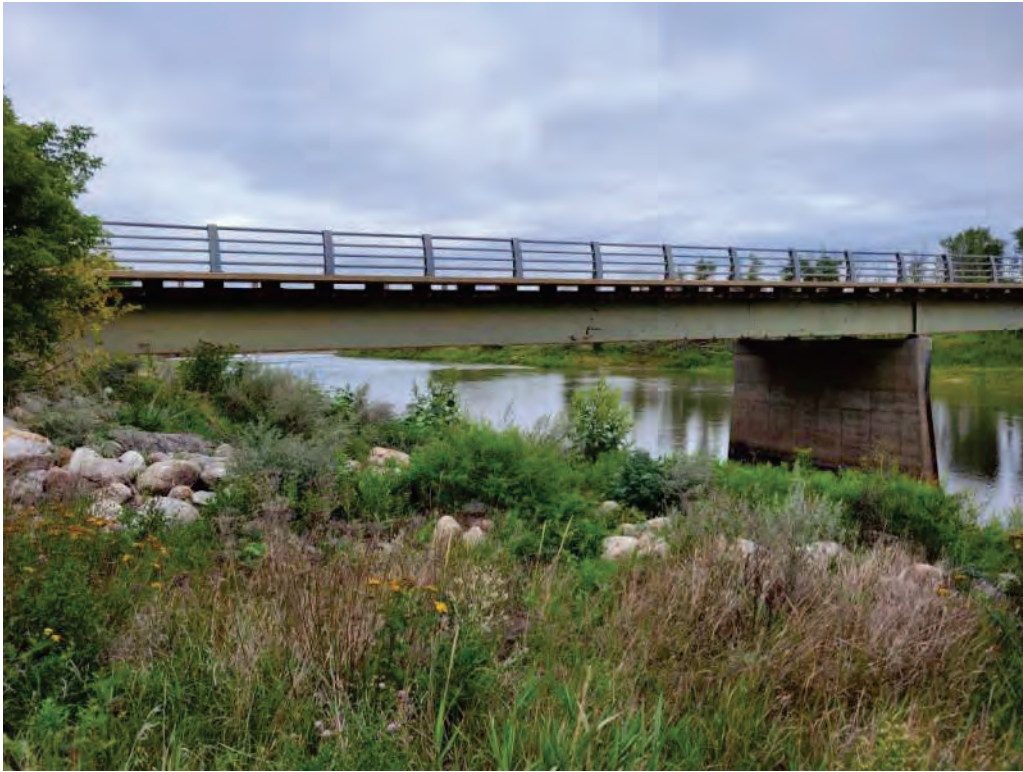
Riprap armouring on north-west side of existing bridge structure occupied by invasive species.
