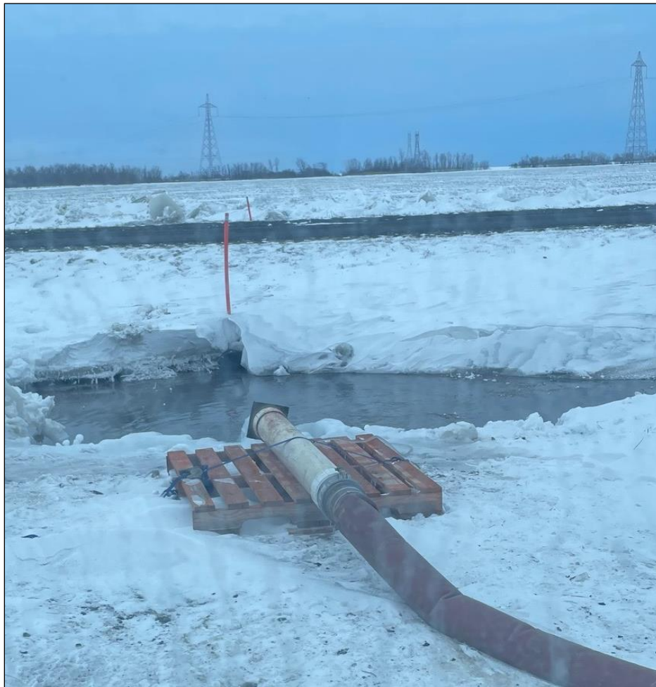
Figure 25 – Discharge Set Up
