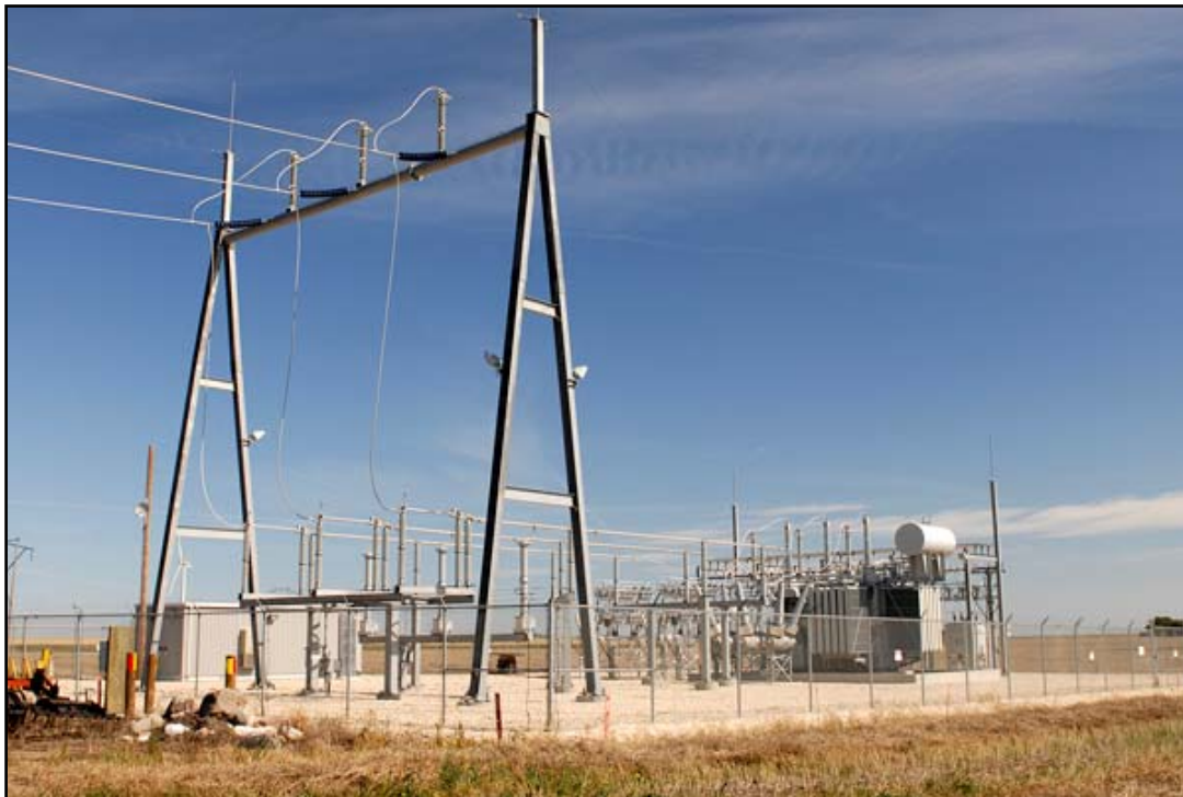
Image 6 – St. Leon Wind Farm Substation
