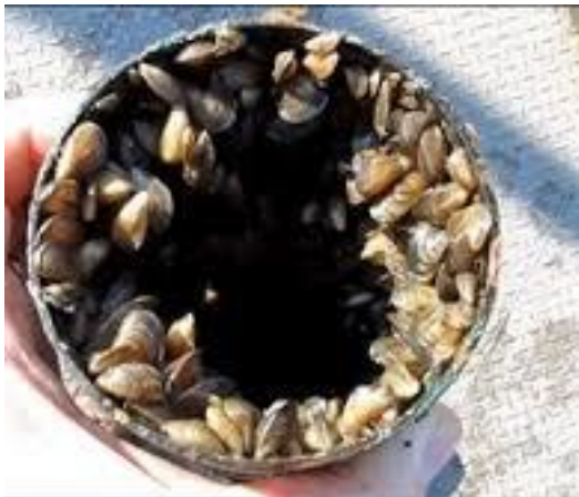
Water intake pipe in Ohio (credit: City of Toledo)
