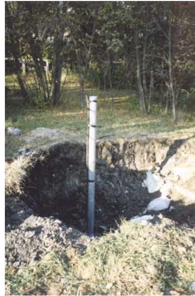
Extension of well casing above grade
