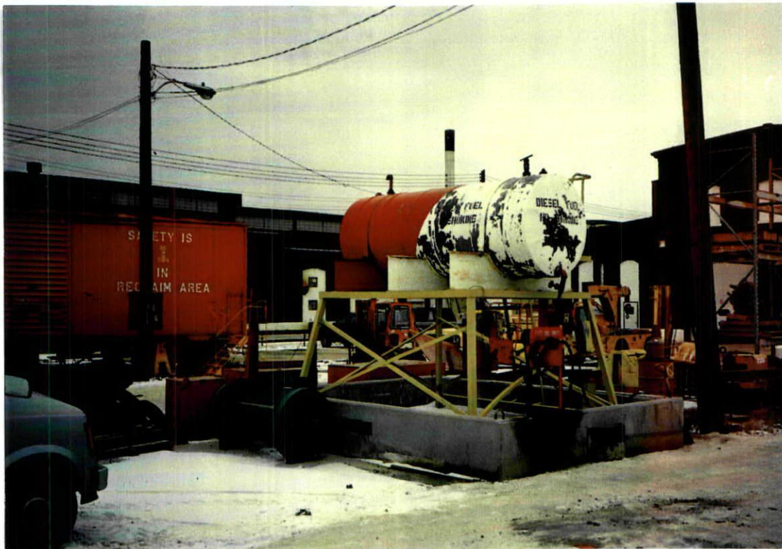
PHOTOGRAPH 3: VIEW OF ABOVE GROUND DIESEL STORAGE TANK LOOKING NORTHEAST. THIS TANK IS LOCATED WEST OF THE MOBILE EQUIPMENT REPAIR FACILITY.
