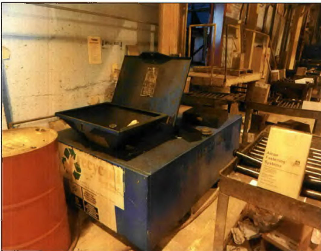
View of used oil aboveground storage tank located in the component shop
