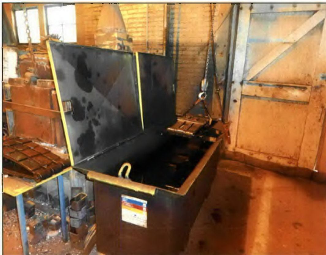
Oil dipping tank located in the welding shop
