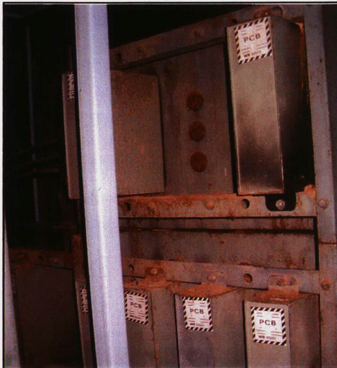
PHOTOGRAPH #19: View of a transformer with 9 banks containing PCBs in Building K.
