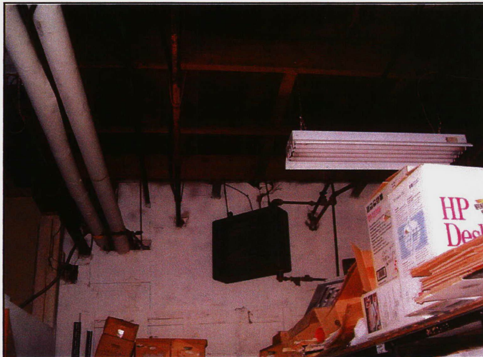
PHOTOGRAPH #7: View of overhead natural gas unit heater in Building E.
