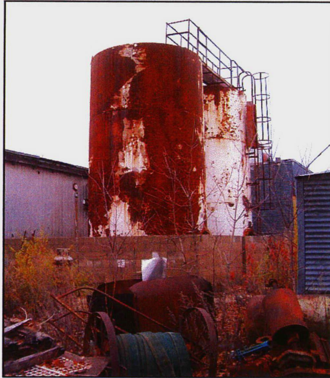
PHOTOGRAPH #43: View of two unused steel tanks at the southeast corner of Building E.
