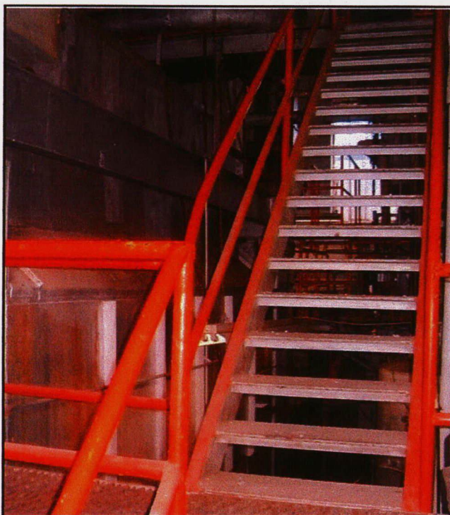
PHOTOGRAPH #13: View of catwalks in the boiler house, Building I.
