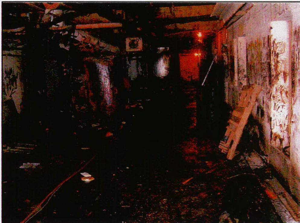
PHOTOGRAPH #10: View of the tar covered concrete floor in the basement of Building E.
