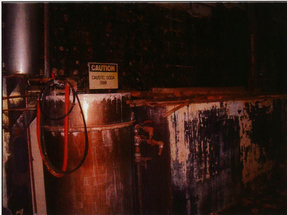
PHOTOGRAPH #20: View of caustic soda tanks in the northwest corner of Building K.
