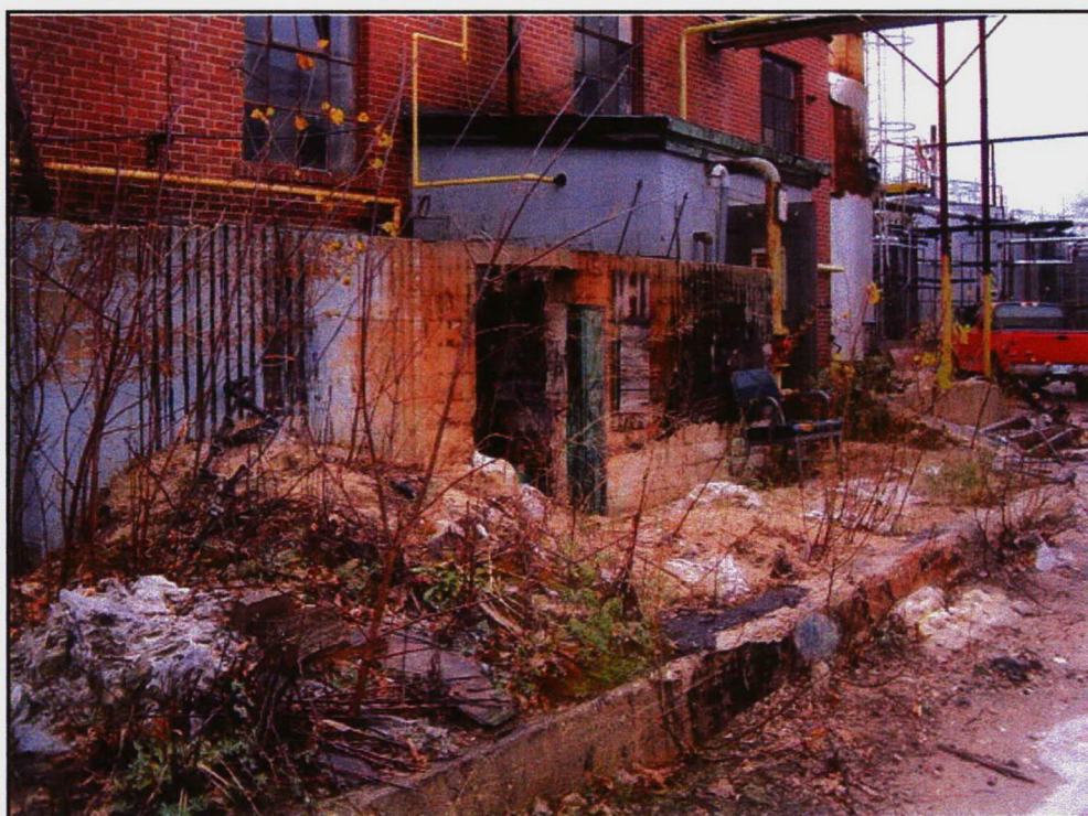
PHOTOGRAPH #42: View of 2 Bunker-C fuel tanks, surrounded by a concrete berm, on the west side of Building I.
