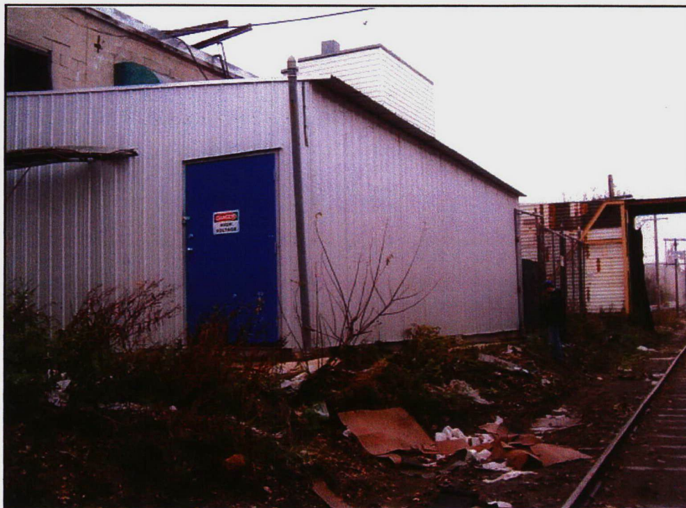
PHOTOGRAPH #41: Metal shed containing 9 transformers adjoining Building K.
