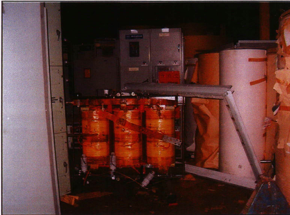
PHOTOGRAPH #11: View of two partial transformers stored in Building E.
