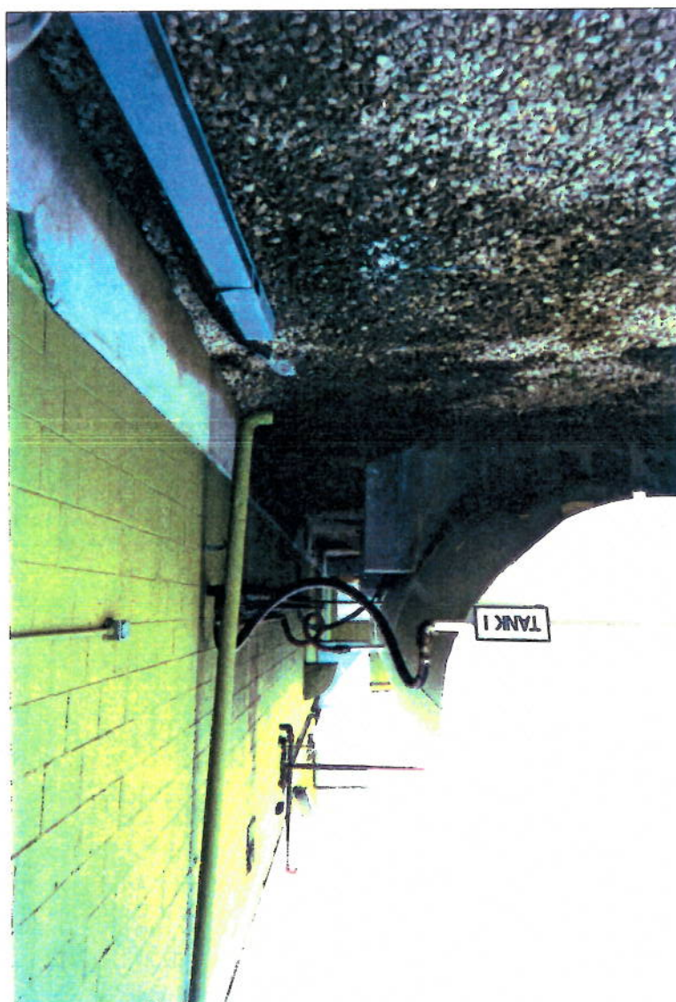
Photo 5 - View of southeast corner of tank compound looking north. MW-4 is located at bottom right corner of photo, at base of Tank 1. Note oil-stained gravel.
