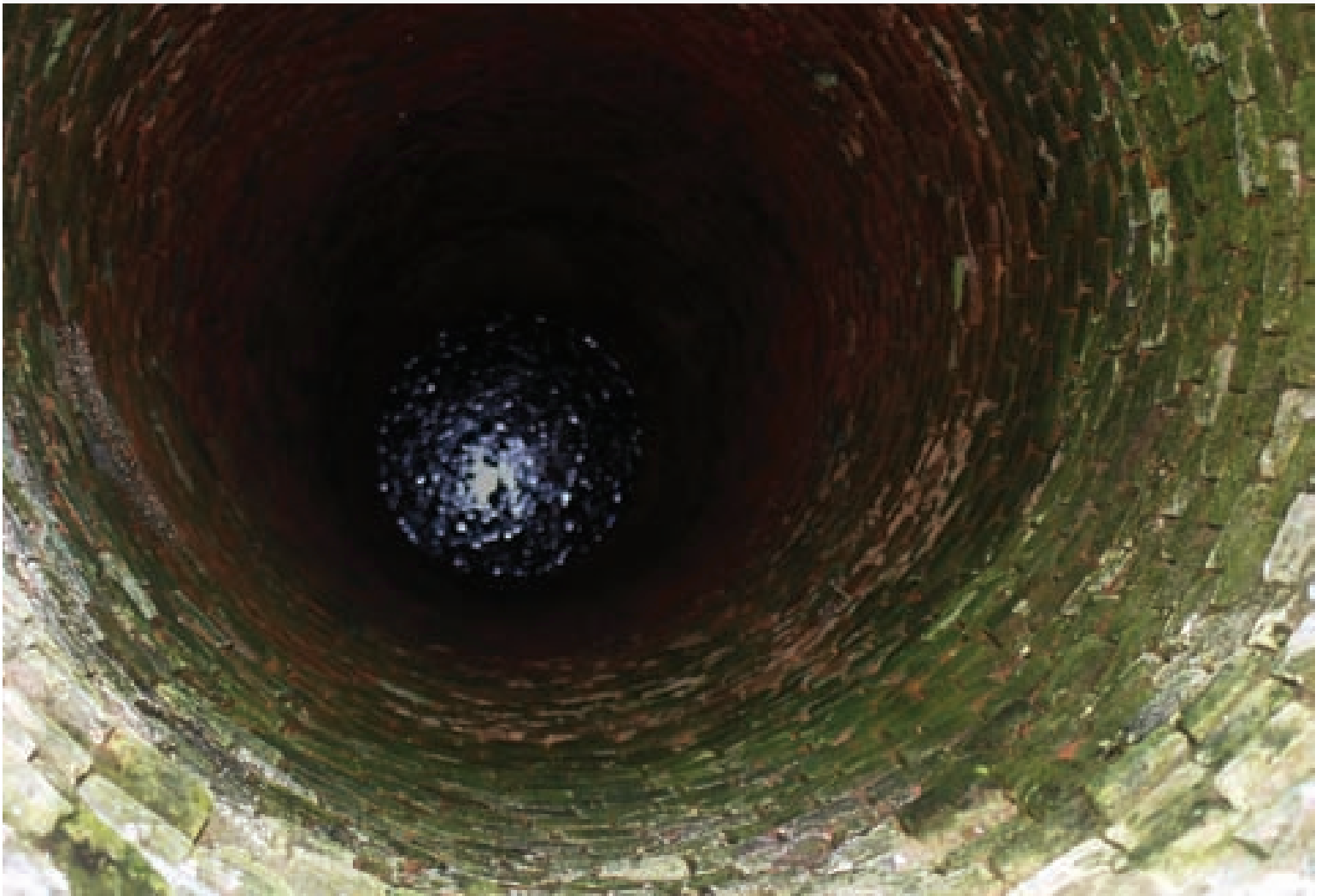
Figure 12: An old, disused well that is about to be sealed. Abandoned or disused wells can act as direct conduits for pollutants at the surface to reach aquifers.
