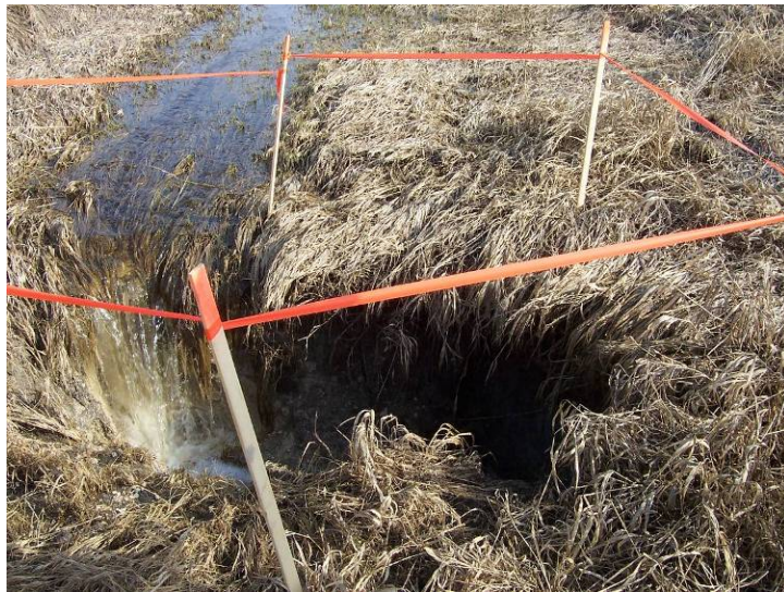
Figure 20: Sinkhole in the Grassmere Drain (2008)
